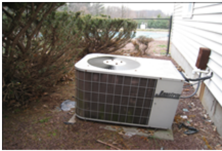
Compressor/condenser unit not level.
