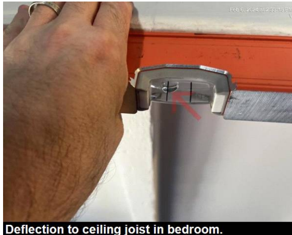
Deflection to ceiling joist in bedroom.
