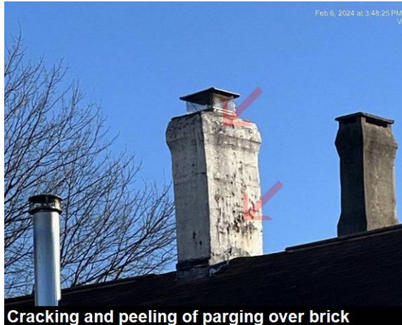
Cracking and peeling of parging over brick
