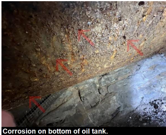
Corrosion on bottom of oil tank.
