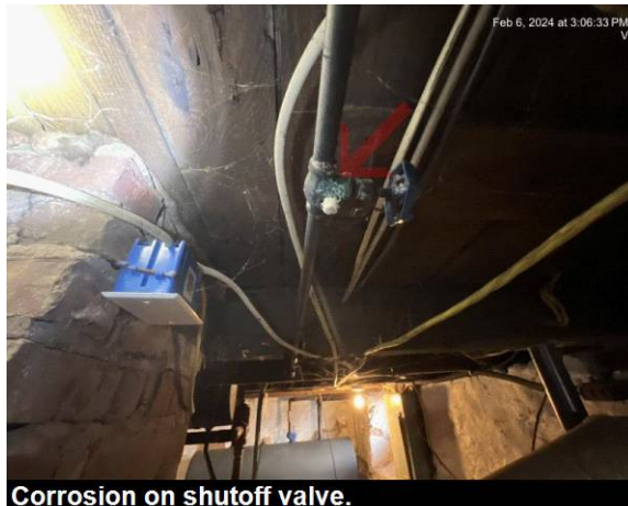
Corrosion on shutoff valve.
