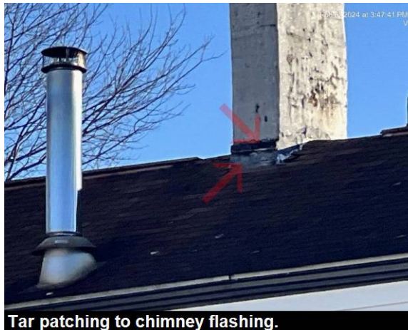
Tar patching to chimney flashing.
