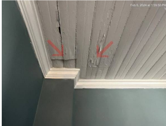
Moisture damage to kitchen ceiling.
