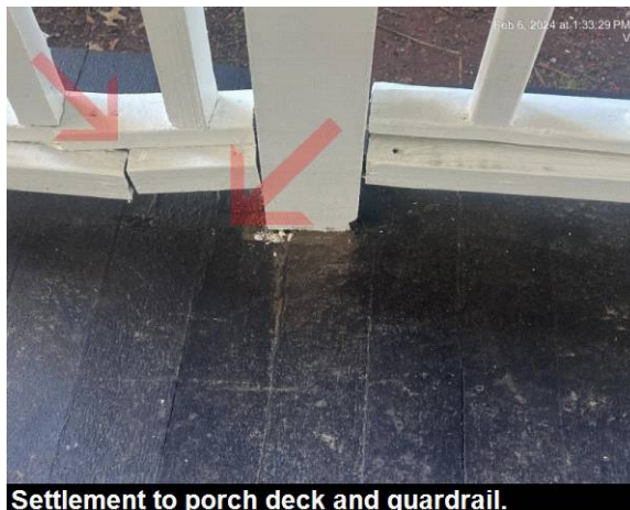
Settlement to porch deck and guardrail.
