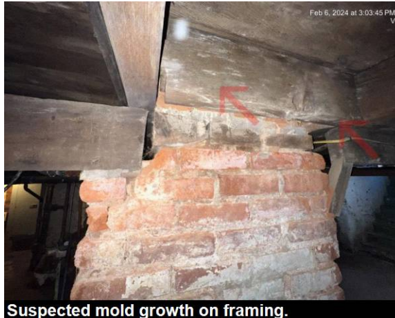
Suspected mold growth on framing.
