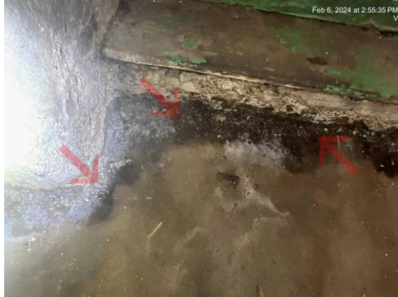
Staining around base of staircase.
