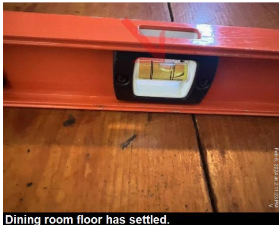
Dining room floor has settled.
