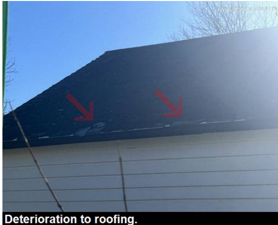
Deterioration to roofing.
