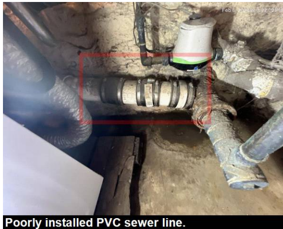
Poorly installed PVC sewer line.
