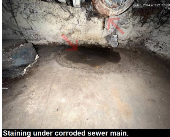
Staining under corroded sewer main.
