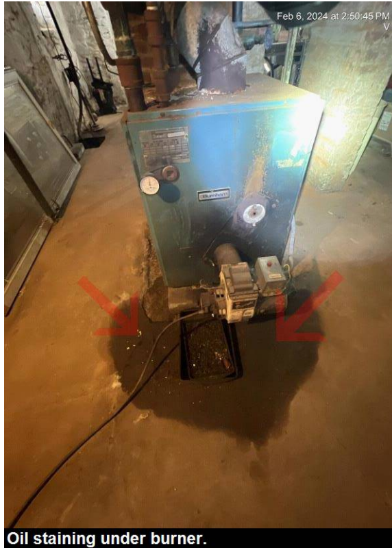
Oil staining under burner.
