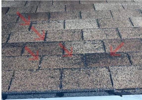
Asphalt granule loss to shingles.
