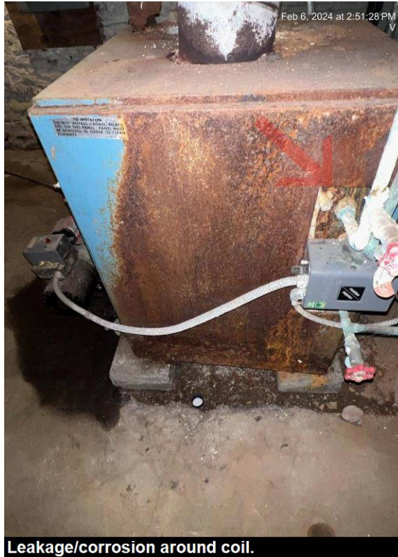
Leakage/corrosion around coil.
