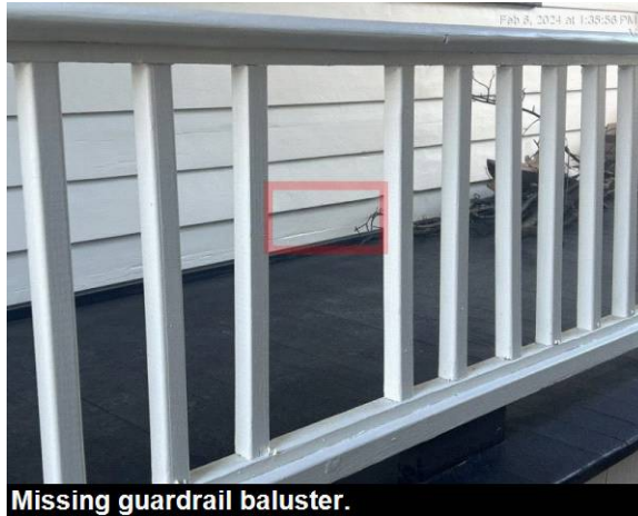
Missing guardrail baluster.
