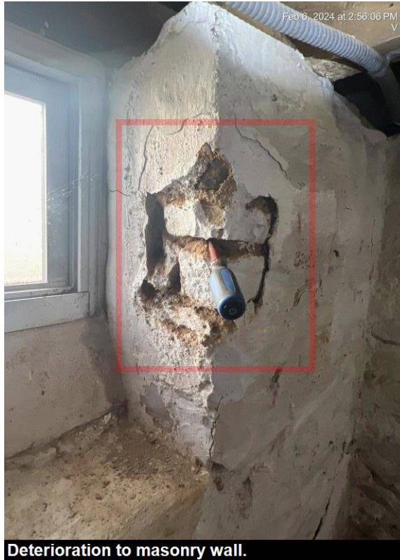
Deterioration to masonry wall.
