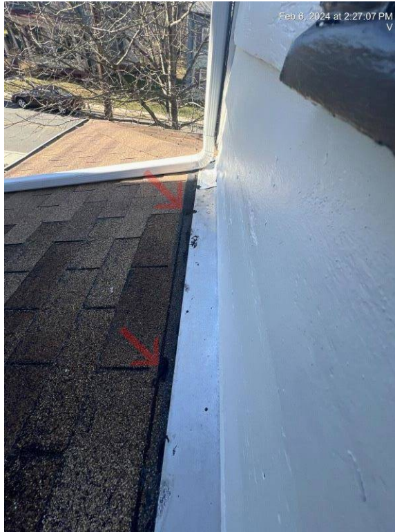
Flashing does NOT cover roofing nails.
