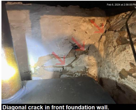
Diagonal crack in front foundation wall.
